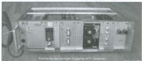
OE7XZR repeater rack
